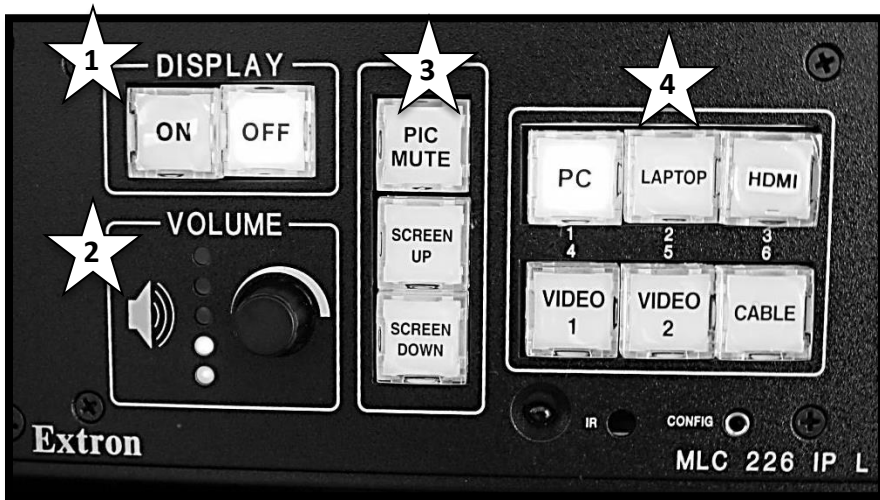
Figure 1: Shows the control panel where Entertainment Center settings are changed.
